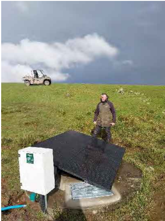
Solar powered pump for livestock watering
